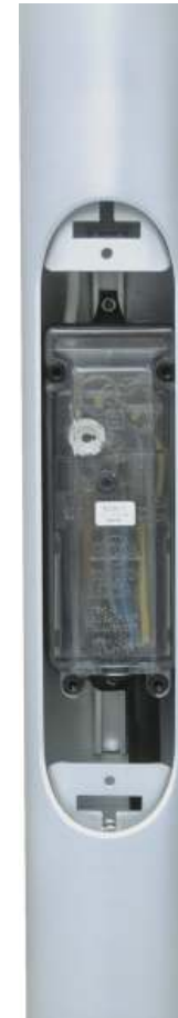
Connection box Installed in aluminium column
